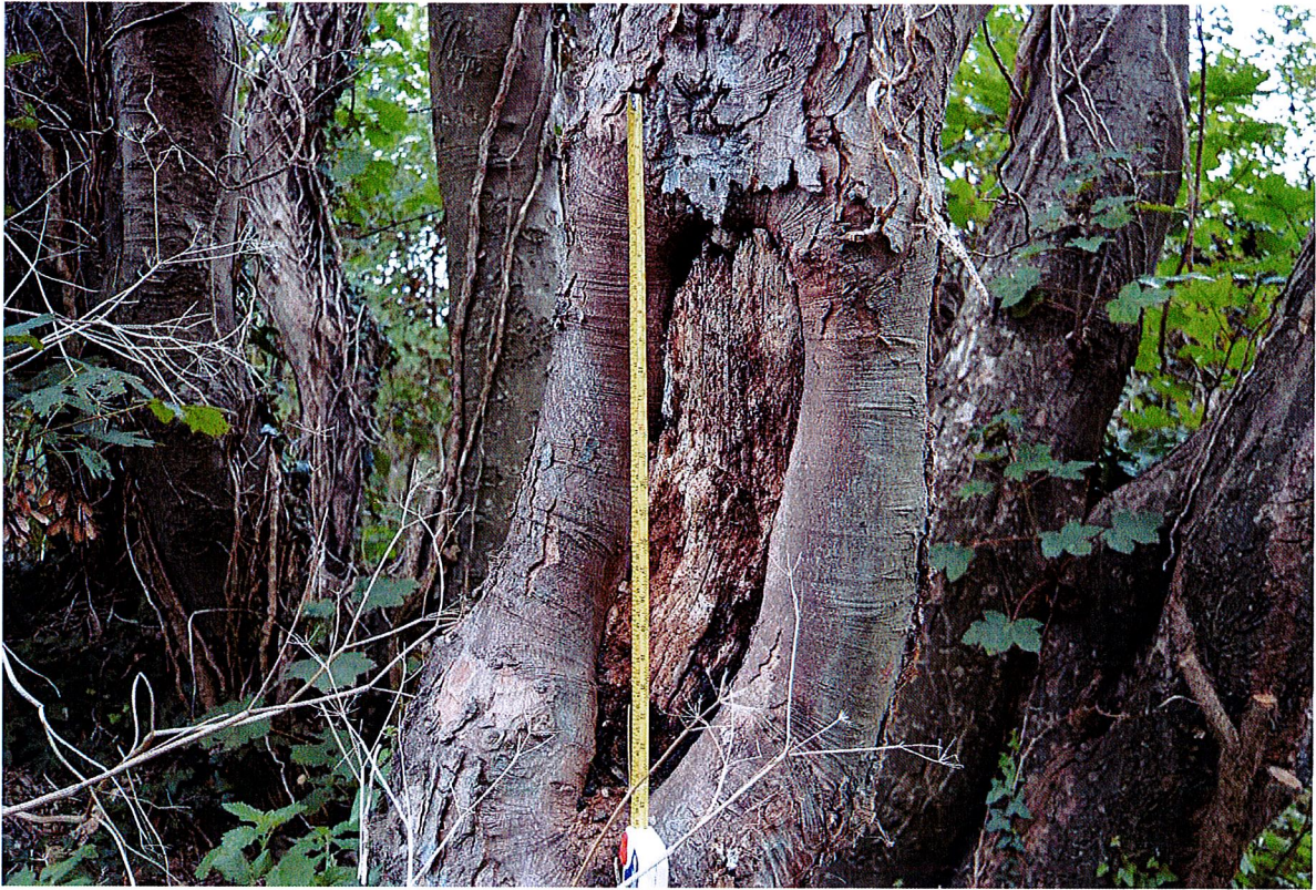
The Copse, area of decay in T26 revealed since Ivy removal.
