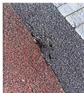
Damage following repairs
