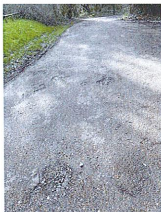
Pot holes in car park
