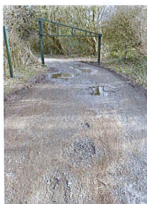
Pot holes at entrance
