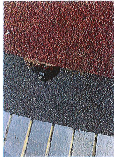
Damaged roundabout surface
