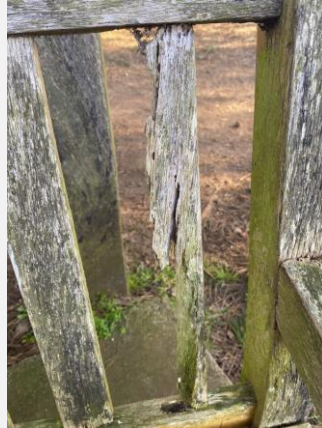
Rotten wooden post
