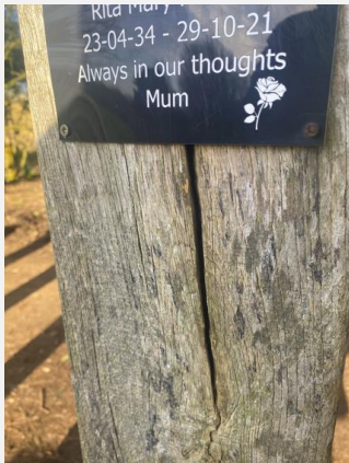
No 13 – crack under plaque & loose
