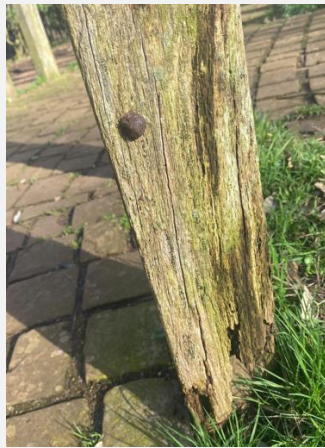
No 30 – rotten at bottom
