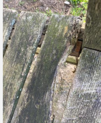
Rotten seating plank
