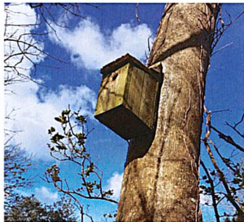
Bird Box number 3, bordering houses at Central Avenue, is rotting by the bird entry hole
